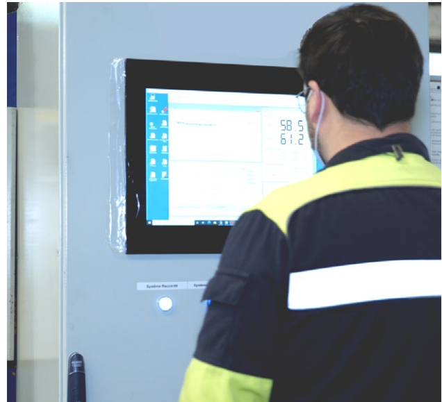
HKL 2 control station
